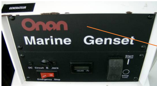
Main breakers for the generator
