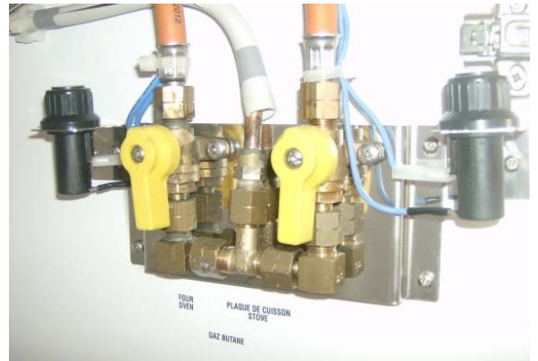
Emergency propane shut off valves below galley sink
