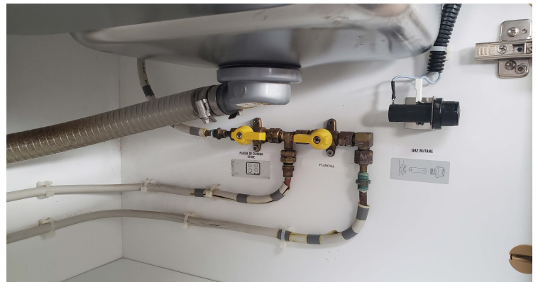
Grill Propane Shut Off valves
